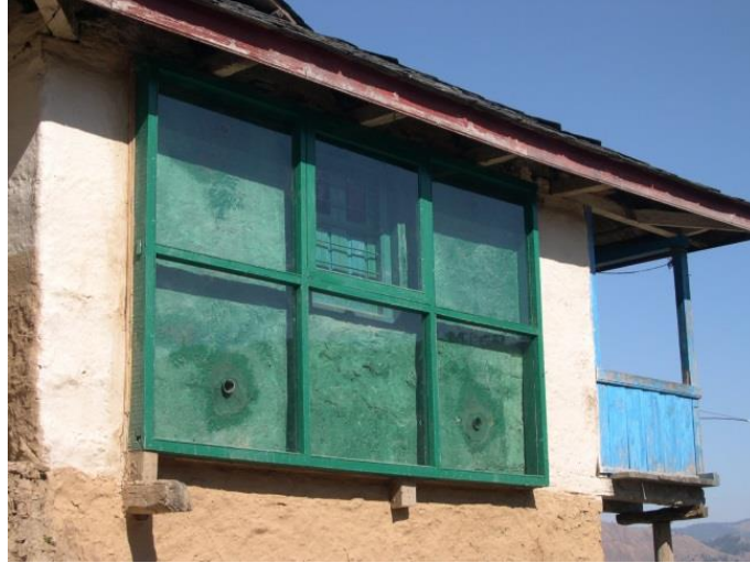
Picture 5. Thermosyphoning air heating panel (TAP) fixed on mud wall
